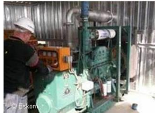
100 kWe diesel genset
